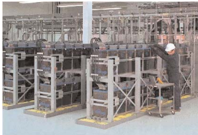
Figure 28. Telecom Back-Up Batteries
