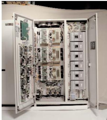
Figure 19. Static Transfer Switch
